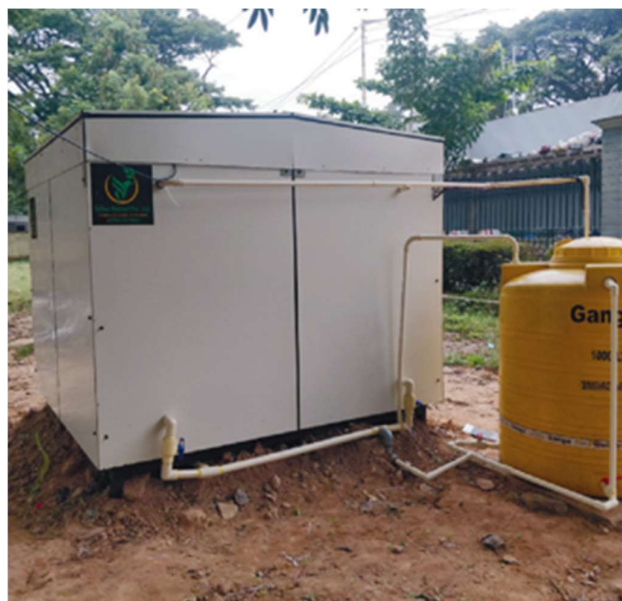
FIGURE 12: R3H2O on-site system installed in open space. Source: Tellus Habitat.
