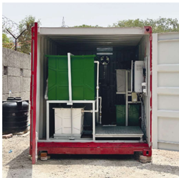
FIGURE 10: Containerized NEWgenerator system. Source: Documentation by UPM GmbH team during a visit to Elefo, 2022.
