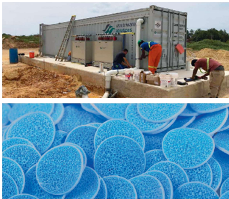
FIGURE 06: Containerized MBBR (top). Biofilm carrier “Mutag Biochips 30TM” used by WTB (bottom). Source: Wastewater Solutions, WTB.
