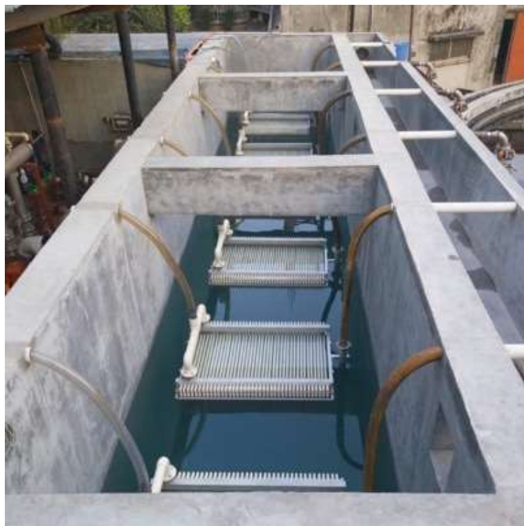
FIGURE 05: View into MBR system with membrane modules. Source: Charm Limited.
